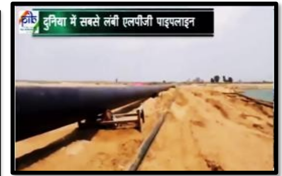
Kandla-Gorakhpur LPG Pipeline Solarizing a total of 158 sites on the country's longest LPG pipeline - spanning 2,757 Kms - from Kandla Port, Gujrat to Gorakhpur, Uttar Pradesh
