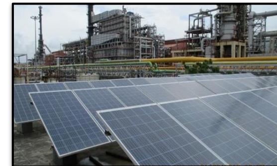
Rooftop Solar Project BPCL (Mahol Refinery)
