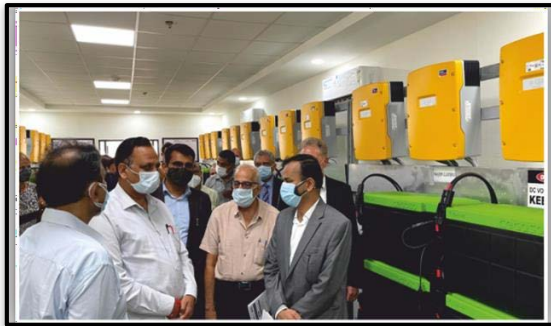
Shivalik Project Micro Grid Solar Power System Installed at Shivalik Grid in Delhi
