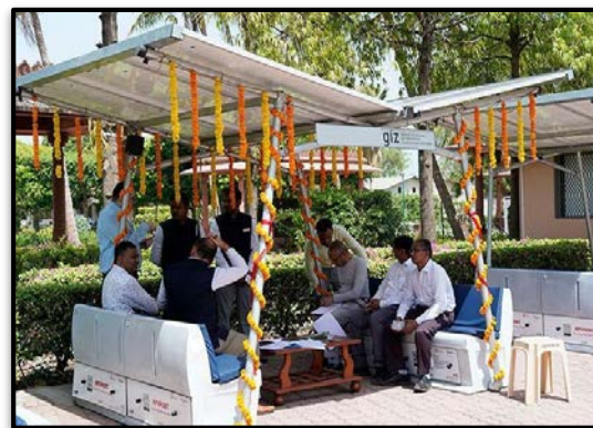
Akshardham Project India's First Portable Rooftop Solar Systems Installed at Akshardham Gandhi Nagar
